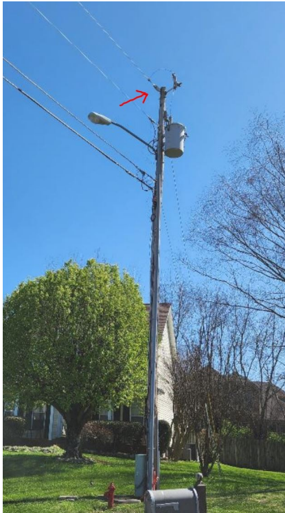
Offending Power Pole
